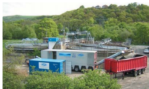
60 m 3 /hr Mobile dewatering system at sewage treatment works
