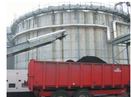
Digetsted sludge dewatering
