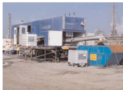
40m 3 /hr rental unit sludge dewatering at a chemical factory
